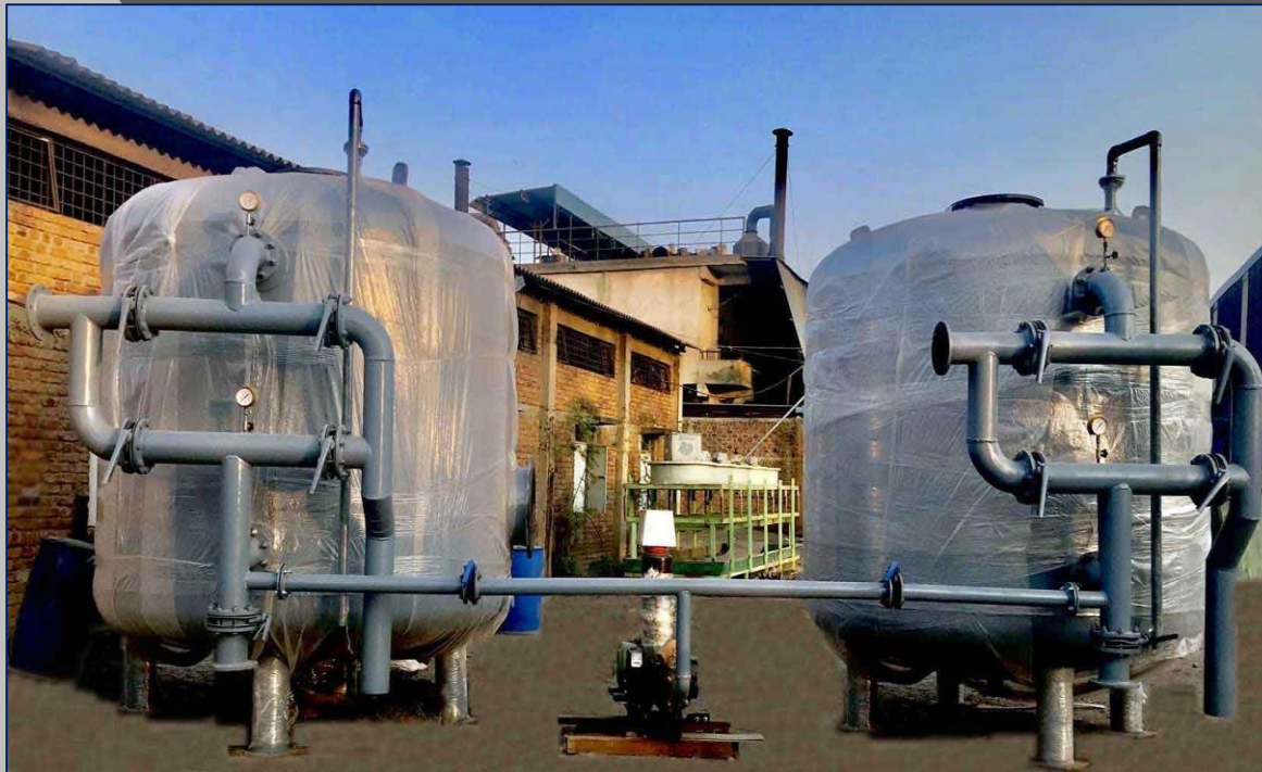
Pressure Sand Filter
